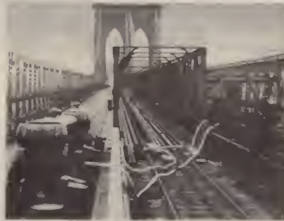
The truss at the outer edge of bridge was built up to the height of inner truss, extreme right.
